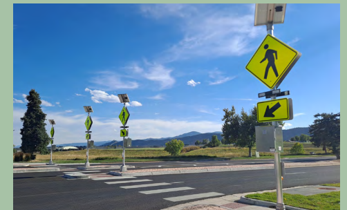
Rectangular Rapid Flashing Beacon (RRFB) in Golden, CO. Source: ITE.
