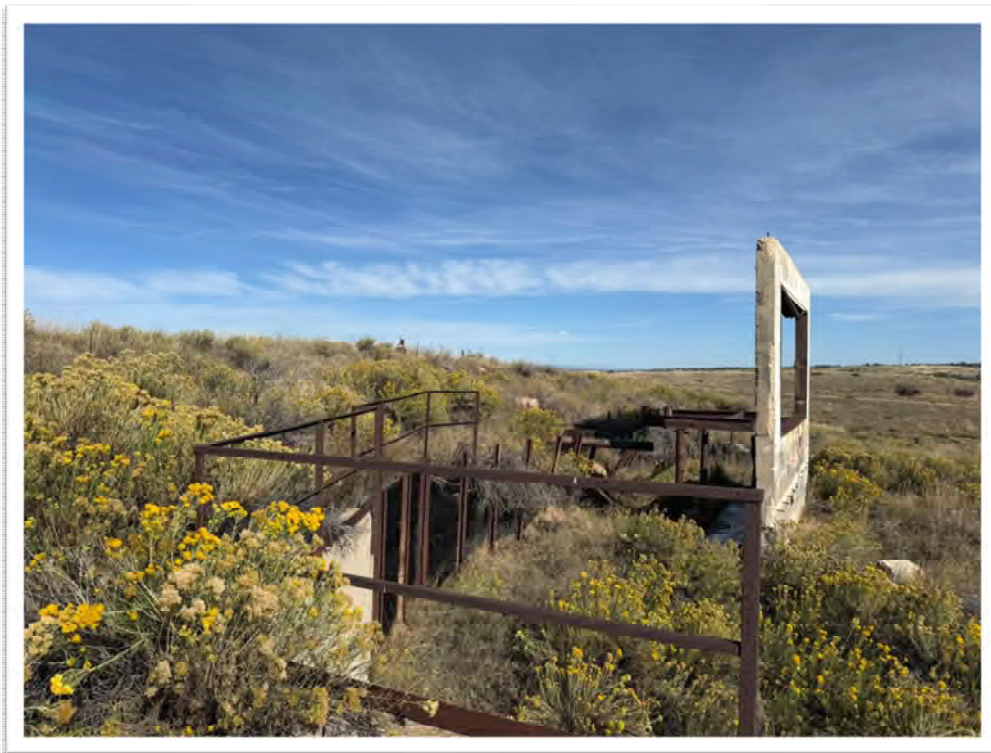
Concrete walls, drains, stairs, various debris adjacent to the eastern boundary (offsite).
